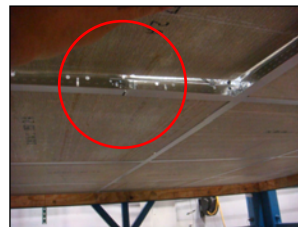
Broken Main Runner Splice (Test#3-250%)
