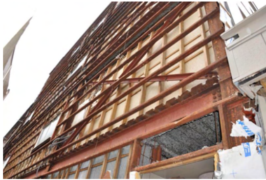
Cladding Wall Damage
