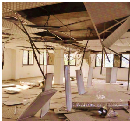
2010 Haiti earthquake: Fixtures installed without safety wires in unbraced suspended acoustical ceiling (photo: Ayhan Irfanoglu, Purdue University).
