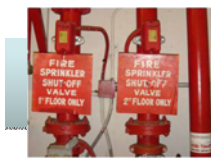
Mechanical, Electrical, and Plumbing (MEP) Components
