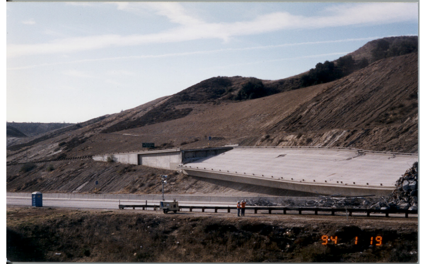
Collapse of Superstructure
