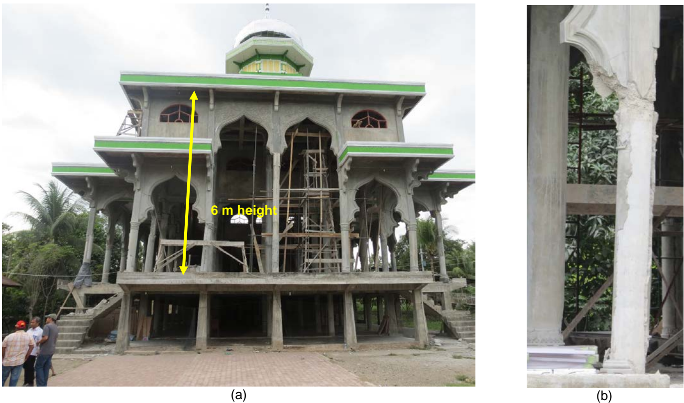
Figure 14. Soft story effect on a mosque structure: (a) overview of mosque with scale, (b) damage to column (photos: Puskim Kemenpupera).
