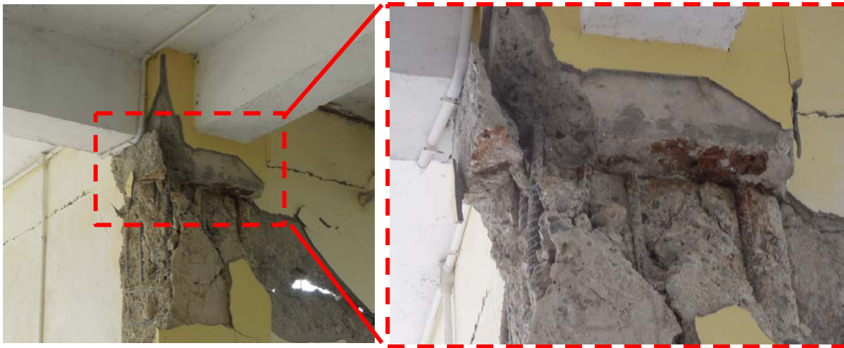
Figure 11. Construction joint failure (photo: Muhammad Riyansyah)
