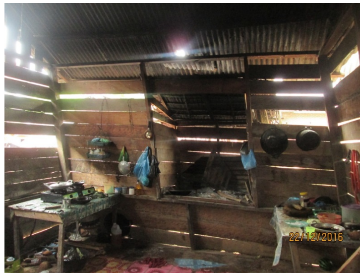
Figure 18. Racking in timber framed house (photo: Build Change).
