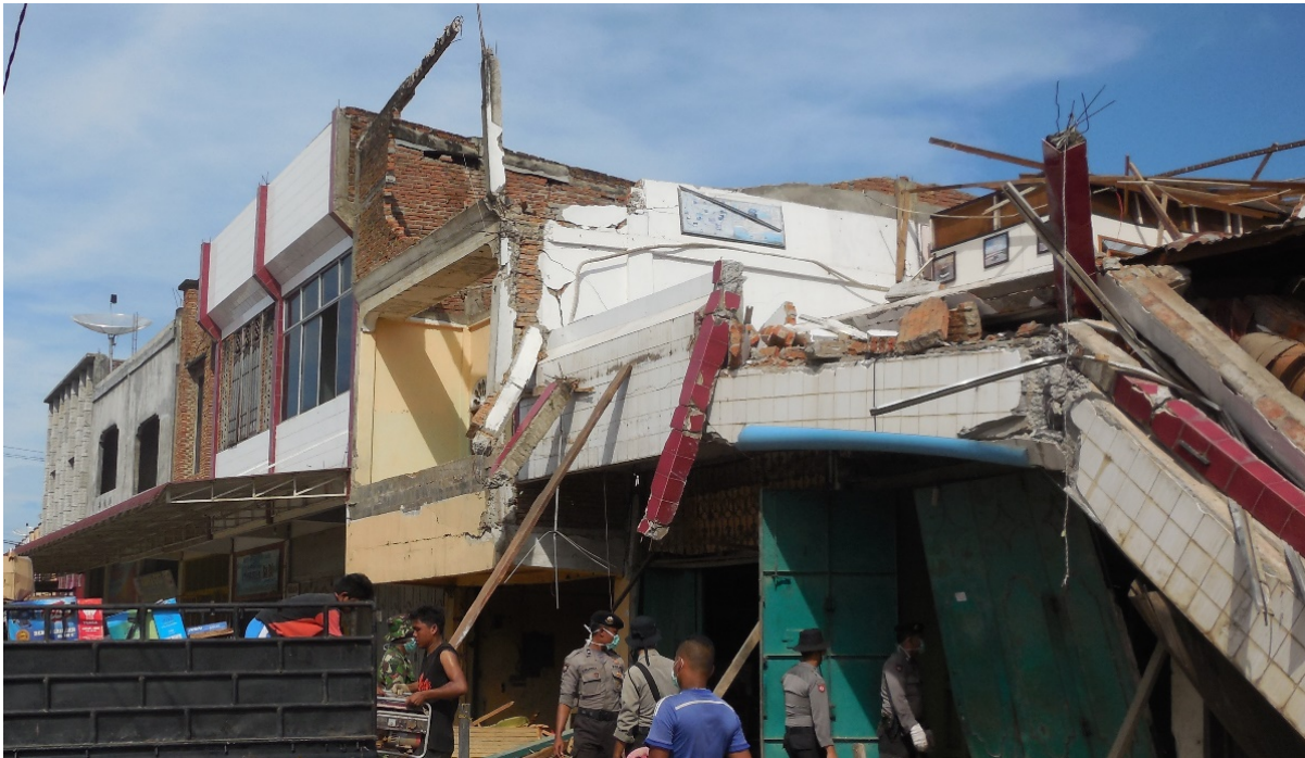
Figure 8. Damages on the some shop-houses that have been modified from existing construction (photo: Muhammad Riyansyah).
