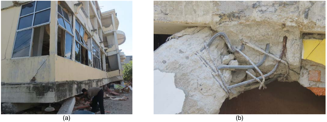
Figure 13. Soft story collapse on a low-rise reinforced concrete building: (a) overview of collapse, (b) mangled rebar due to collapse (photos: Puskim Kemenpupera).
