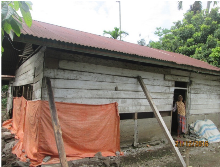
Figure 19. On-grade timber house with partially collapsed skirt wall (covered by tarp) (photo: Build Change).
