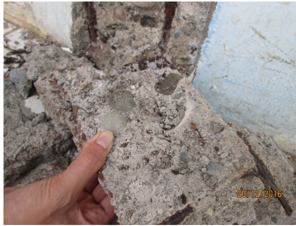
Figure 24. Low quality concrete in school column (photo: Build Change).
