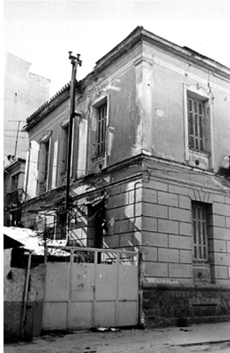
Fig. 7 Slightly damaged, 2-storey masonry building (GREEN)
