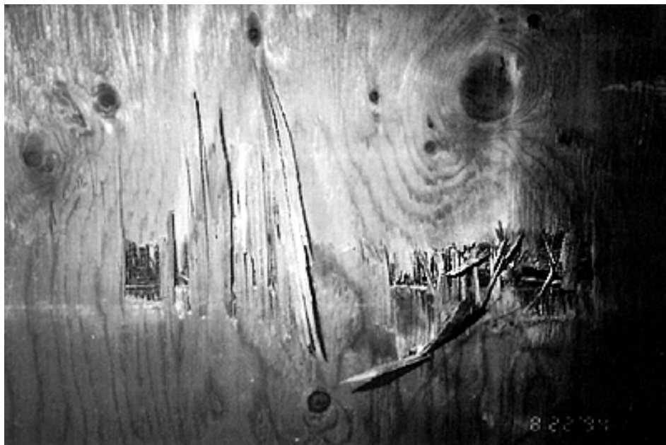
Fig. 14 Local damage to plywood shear wall (YELLOW)
