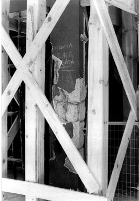
Fig. 3 Emergency support due to failed column
