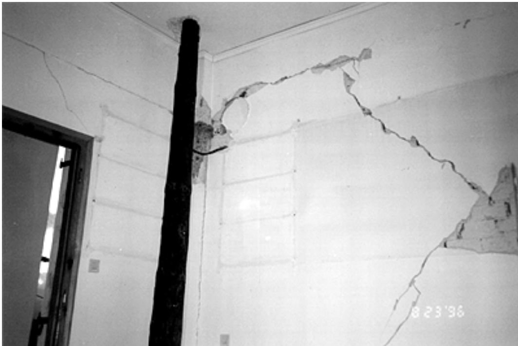
Fig. 24 Severe cracking of several interior brick infill walls in a R/C building (YELLOW)
