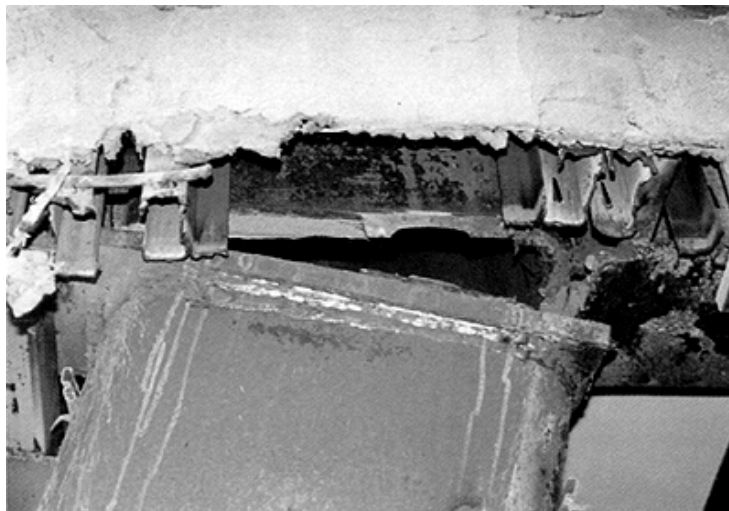
Fig. 32 Fractured weld of the panel plate in beam - column joint (YELLOW)
