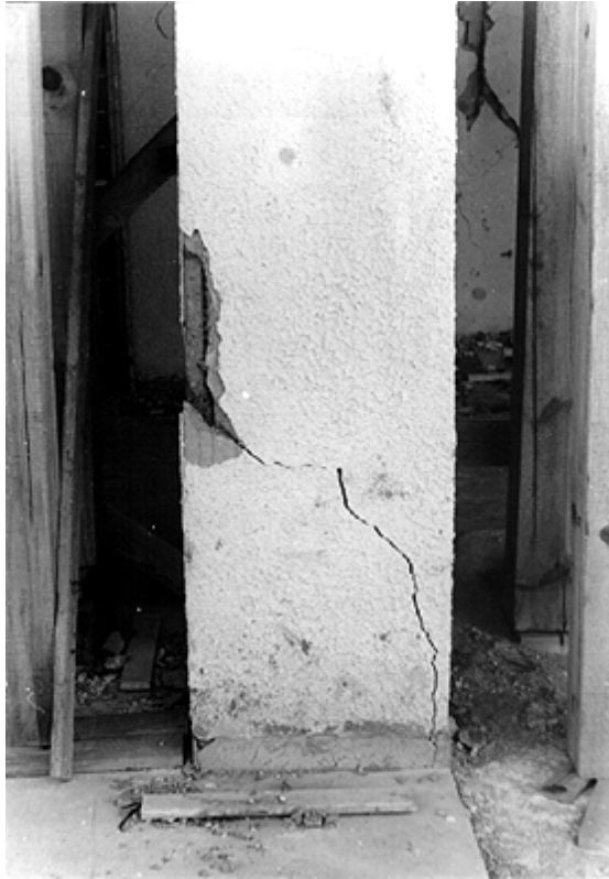
Fig. 23 Fracture of one column (others OK) and several cracked infills of a R/C building (YELLOW)
