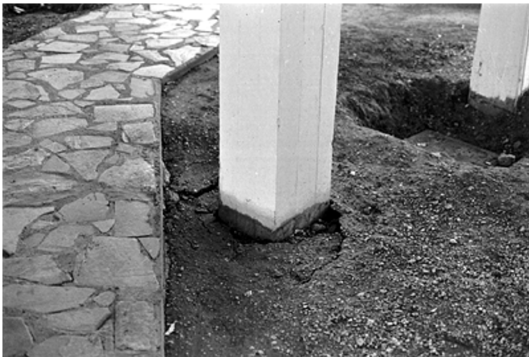
Fig. 27 Ground problems accompanied by heavy structural damage in R/C columns (RED)
