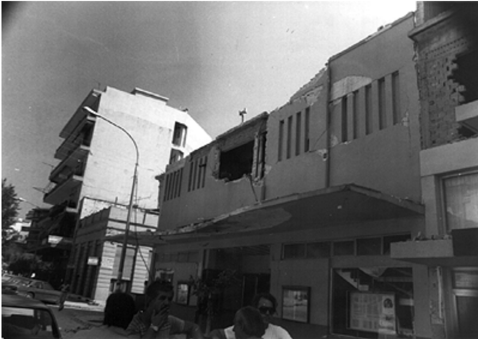
Fig. 1 Partially collapsed wall and parapet, requiring urgent demolition
