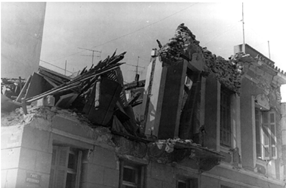
Fig.2 Hazardous, partially collapsed masonry building requiring urgent demolition
