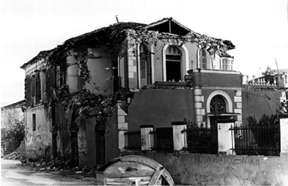
Fig. 11 Partial collapse of masonry building (RED)
