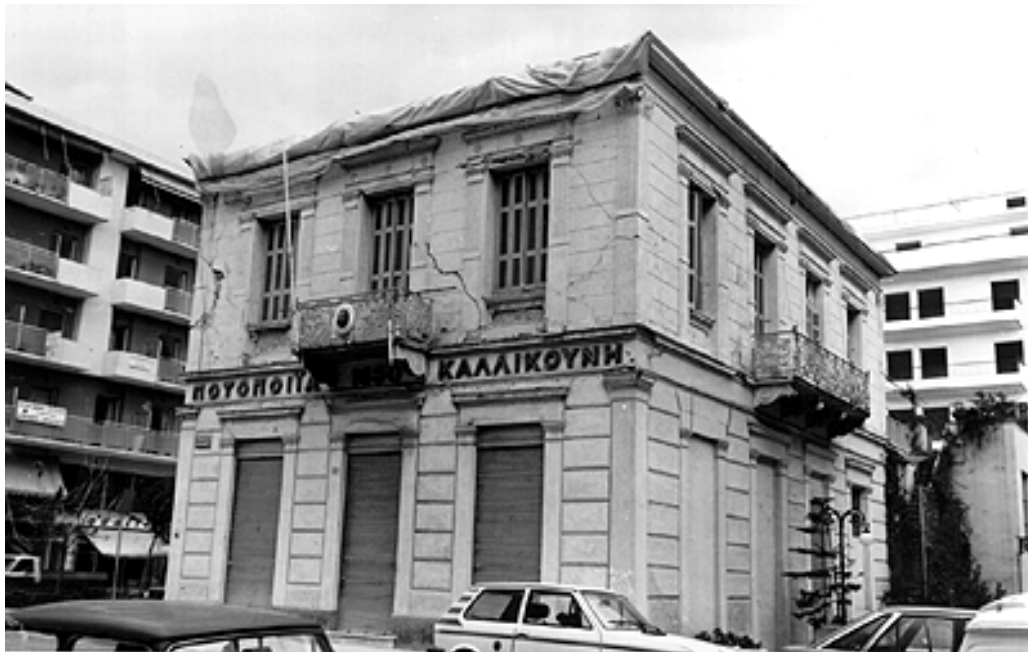
Fig. 8 Moderately damaged, 2-storey masonry building (YELLOW)
