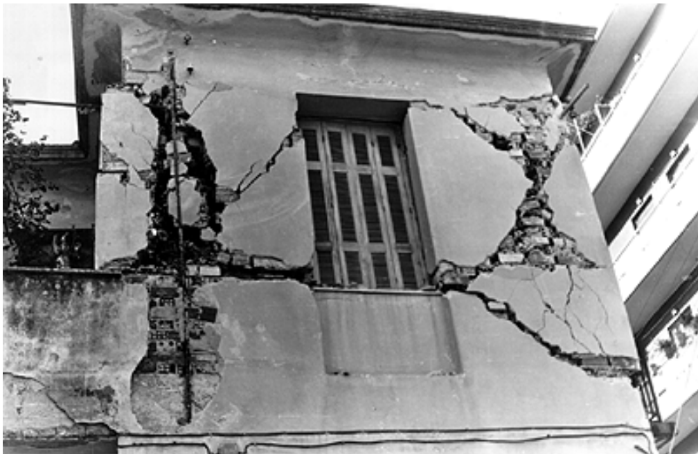
Fig. 10 Severe damage of masonry building (RED)
