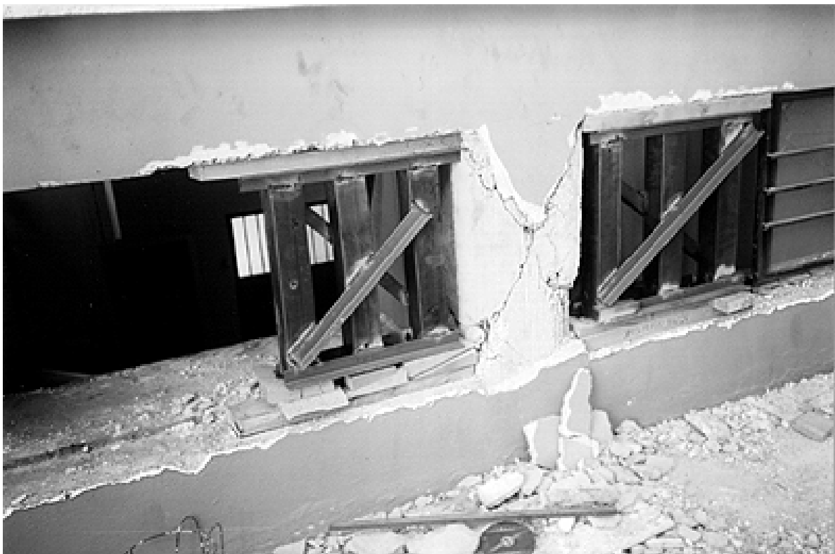
Fig. 22 Local heavy damage in short columns of R/C building (YELLOW)
