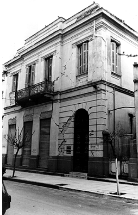
Fig. 9 Moderate to heavy damage of 2-storey masonry building (YELLOW)
