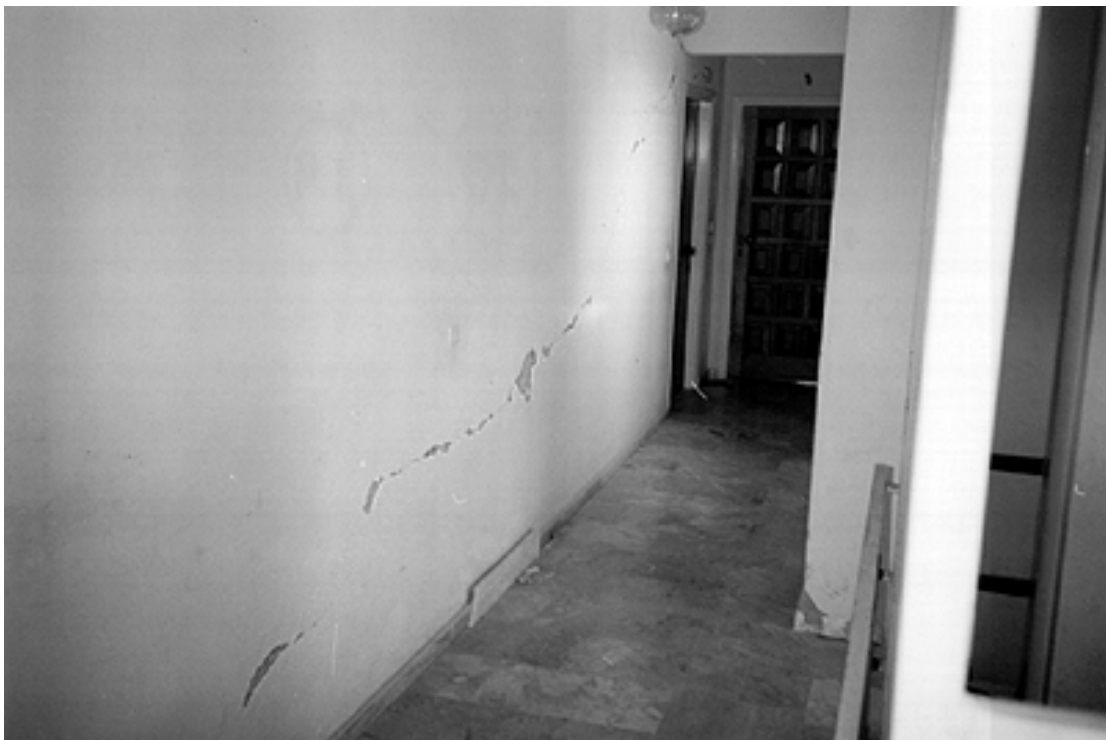
Fig. 20 Minor cracking in brick infills of R/C building (GREEN)
