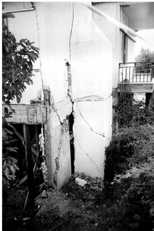
Fig. 26 Crashed R/C columns (several) and dislocation of building (RED)
