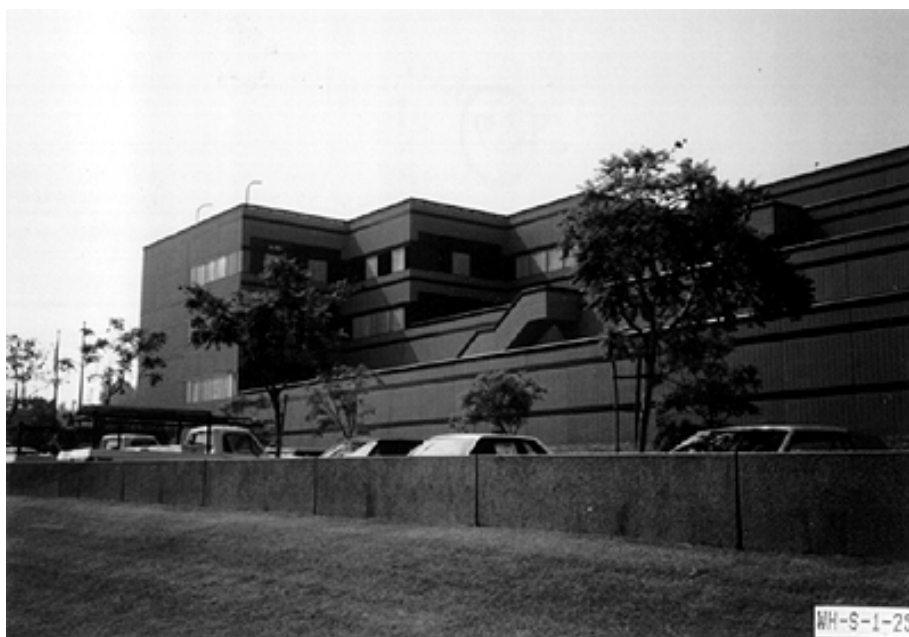
Fig. 29 Four story steel building with extensive broken glass and several buckled braces (YELLOW)
