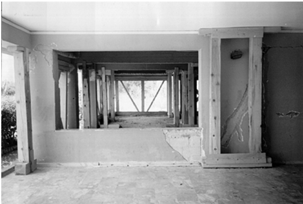
Fig.4 Emergency support of damaged, open ground story, of concrete building
