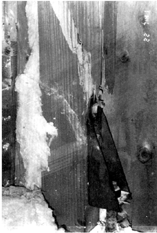
Fig. 15 Fractured post above the holddown (YELLOW)
