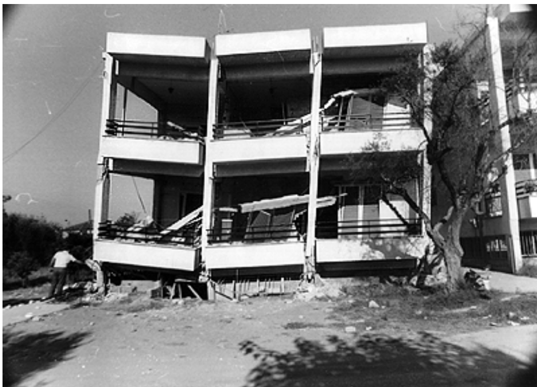
Fig. 28 Ground story collapse and tilt of a 2 ½ story R/C building (RED)
