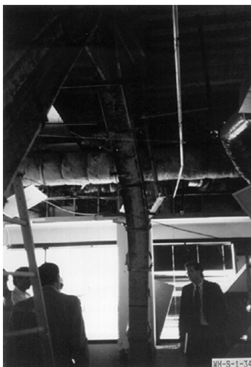
Fig. 30 Buckled brace of building in Fig 29
